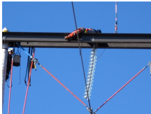
Picture 3 Transmission Line Maintenance Technician on the top of FRP Cross arm installing hardware on live (energized) line
